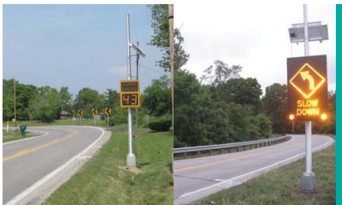
Figure 4. Two Examples of Installed DCWS (MTC 2009)
