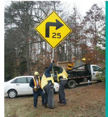
Figure 7. LED-Enhanced Curve Warning Sign, KY 82 (Image: KYTC)
