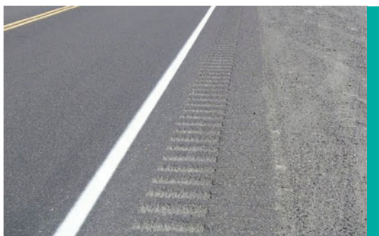
Figure 18. Sample of Installed SRS in Washington State (FLG 2014)
